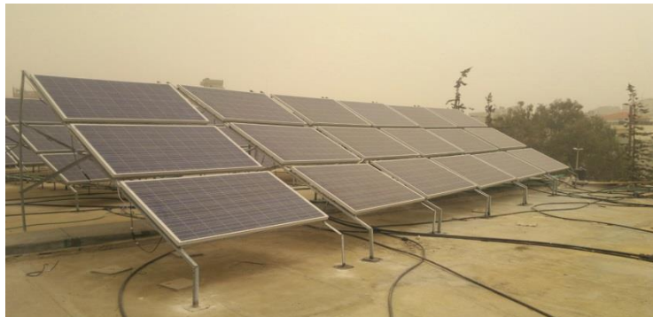
Figure 2.6: Solar energy project in Al-Naser hospital
