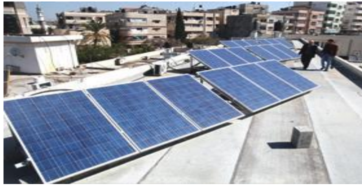
Figure 2.7: Solar energy project in Al-Shifa hospital
